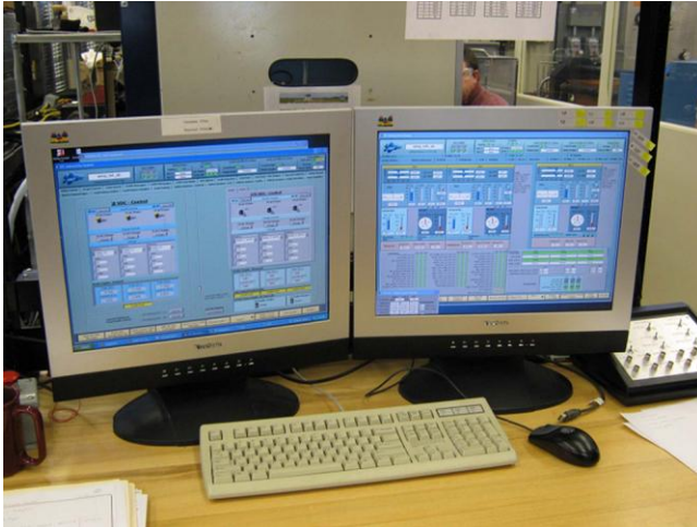
Figure 8. Integrated test computer (ITC)
