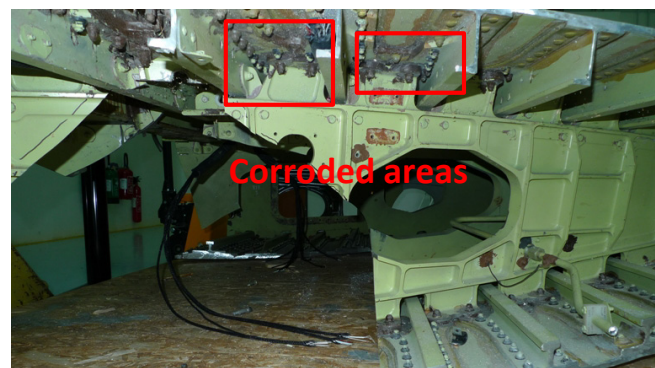
Figure 14. A320 wingbox with corrosion flaw inside the wing. (Acknowledgments to Airbus and EADS-IW)
